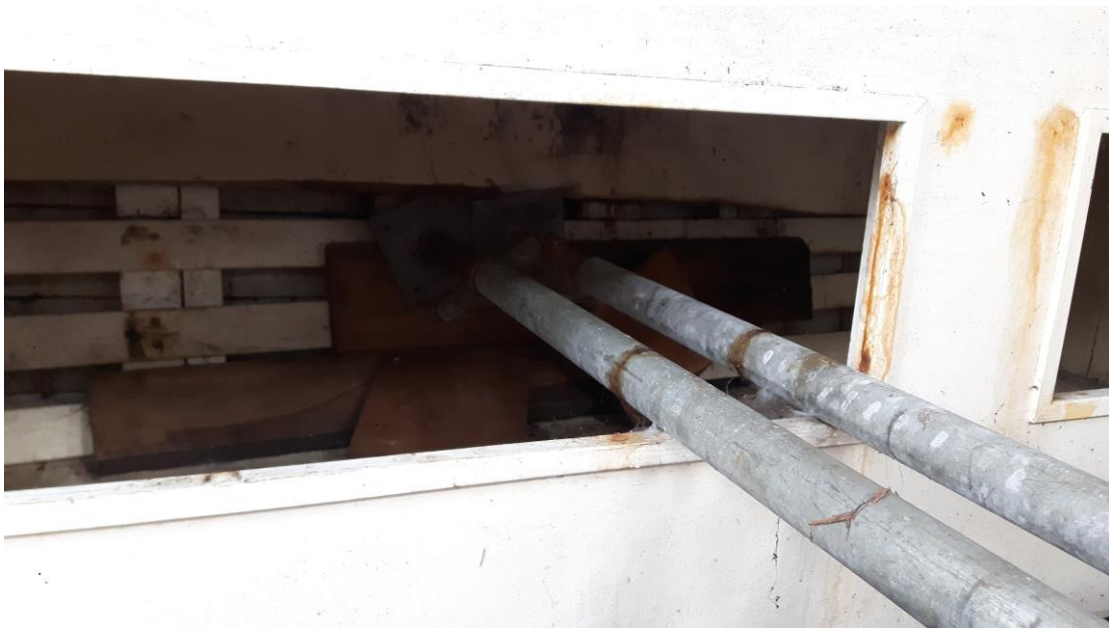
Aft cabin, scaffolding poles – possibly left from last maintenance period
