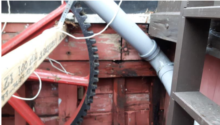
Engine room Aft Starboard, rotten beam shelf and rotten beam shelf stringer
