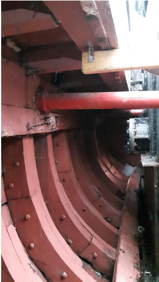
Framing in the engine room, rotten bilge stringer, rotten beam shelf, rotten beam shelf stringer
