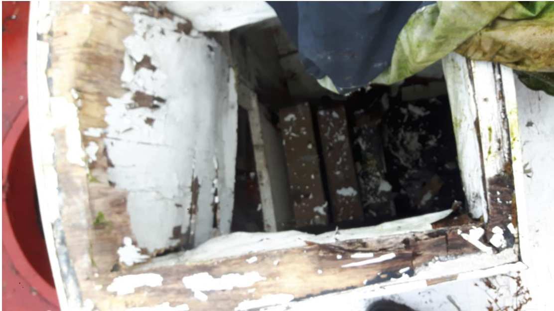
Aft cabin rotten collapsed deck head
